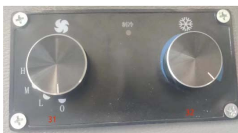
Figure 2-22 Air conditioning control panel
